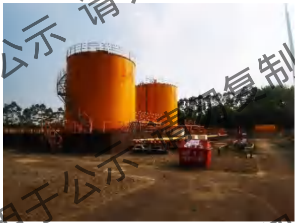
油罐、围堰、消防沙箱
