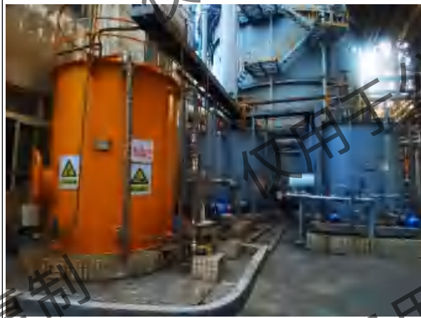
湿式除尘器碱液罐
